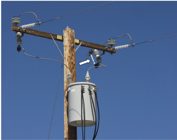
Figure: Pole-mounted secondary distribution transformer with its OC fuse (shown with a white arrow)
